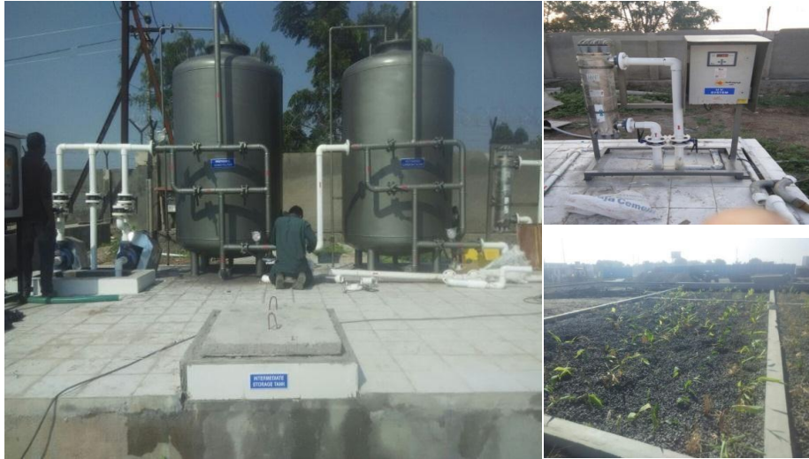
Sara Builders & Developers Pvt. Ltd. - 500 CMD STP
